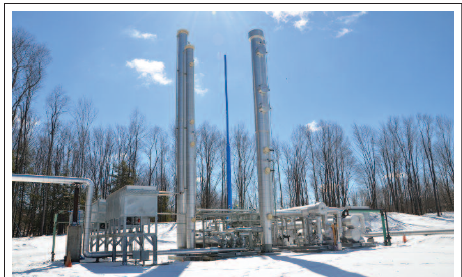
The Refrigerated Joule-Thompson plant developed by Joule Processing can take natural gas temperature to minus 145 degrees with 90 percent propane recovery. The company says the JT plant is a "faster and less expensive" alternative to cryogenic plants. They can be sized anywhere from 5 million to 100 million cubic feet a day. This JT plant in Union City, Pa., has a capacity of 15 MMcf/d.
