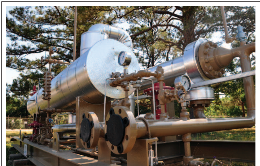
Joule Processing says it takes pride in working with customers to come up with the best solutions for their applications. This 5 million cubic foot a day Joule-Thomson plant is in service for Petrohawk Energy Corp. in the Eagle Ford Shale. It is one of four standard-size J-T plants for hydrocarbon dew point control, Joule reports, adding that the skid can be loaded on a flatbed truck.
